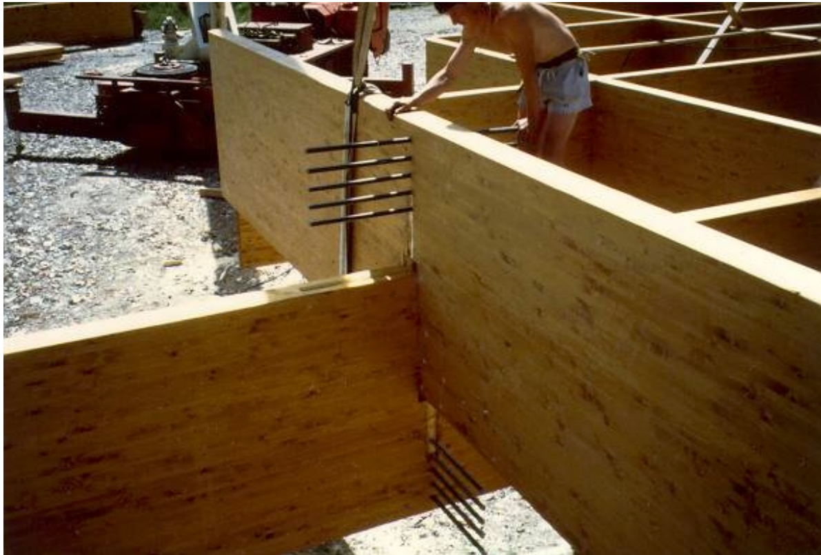
Figure 2 - Typical applications in new construction. Glued-in rods for glulam structures at “L’Aquilone di Chicco” (Grandate - CO). Design: Geom. Giovanni Cenci. Works: Holzbau spa. Scientific advice: Prof. Piazza, Università di Trento.
