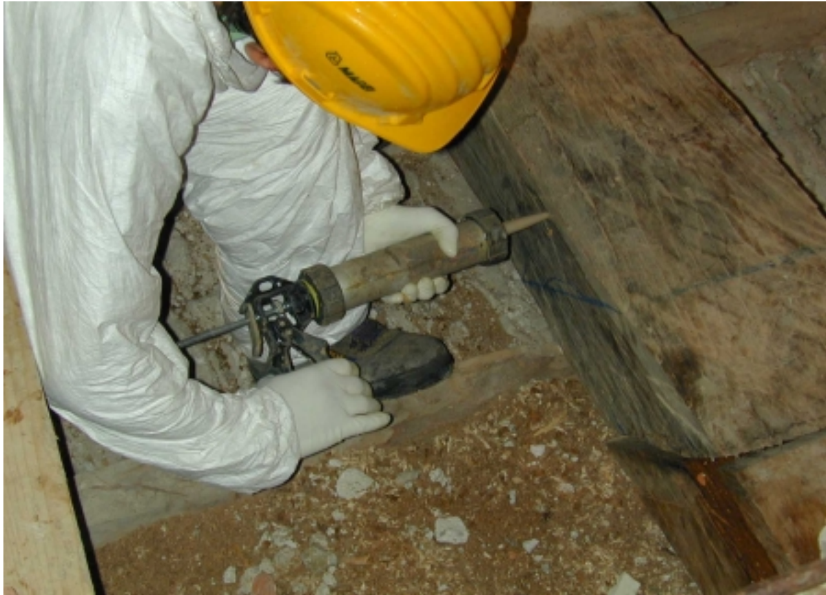
Figure 1 – Typical applications in restoration. Glued-in rods for the substitution of rotten heads of Oak beams at "Poggio Cusiano" (Miasino - NO). Design: Arch. Daniele Scalcon. Works: LegnoPIÙ snc. Scientific advice: IRL/CNR.
